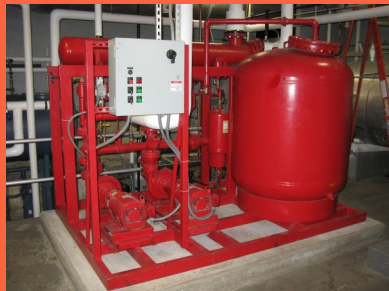
B&G Heat Transfer Package installed at Carteret High School.
